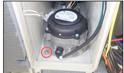
Fig. 10. Circulation pump screw location.
