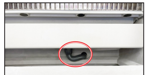
Fig. 6. Sump drain fitting location.
