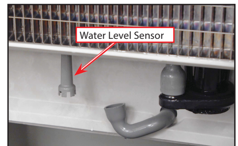
Fig. 2. Water level sensor location. Sump tank removed for illustration.
