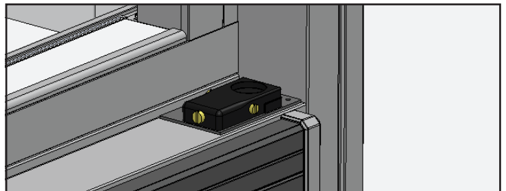
Fig. 27. Correctly installed replacement torque master assembly.
