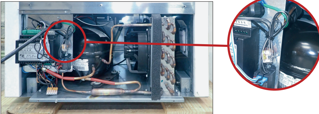
Fig. 4. Remote alarm contact location.
