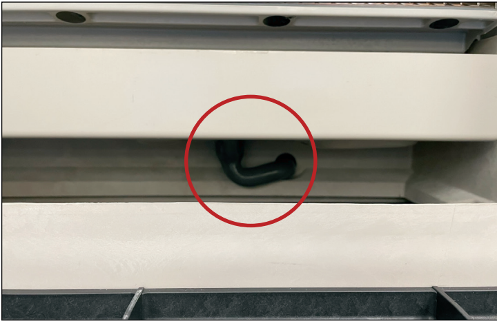
Fig. 2. Sump drain fitting locations.
